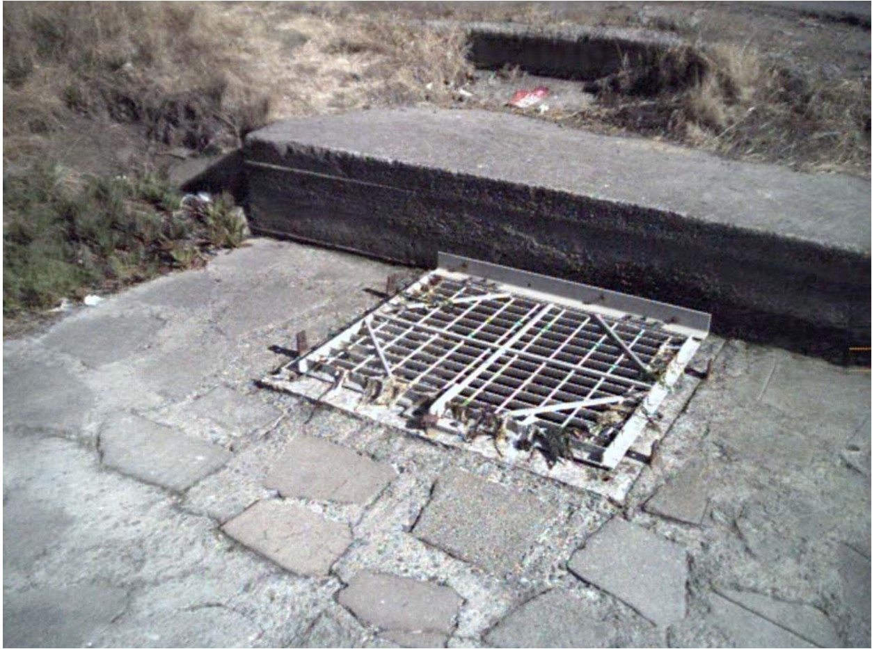
Figure 2-10. Grate Over Weir Box in the Connection Between the Model Yacht Basin and the Potter Street Stormdrain
