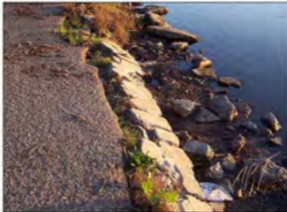
Figure 52: Rock Wall Falling off Shoreline Trail on East Shore of Main Lagoon
