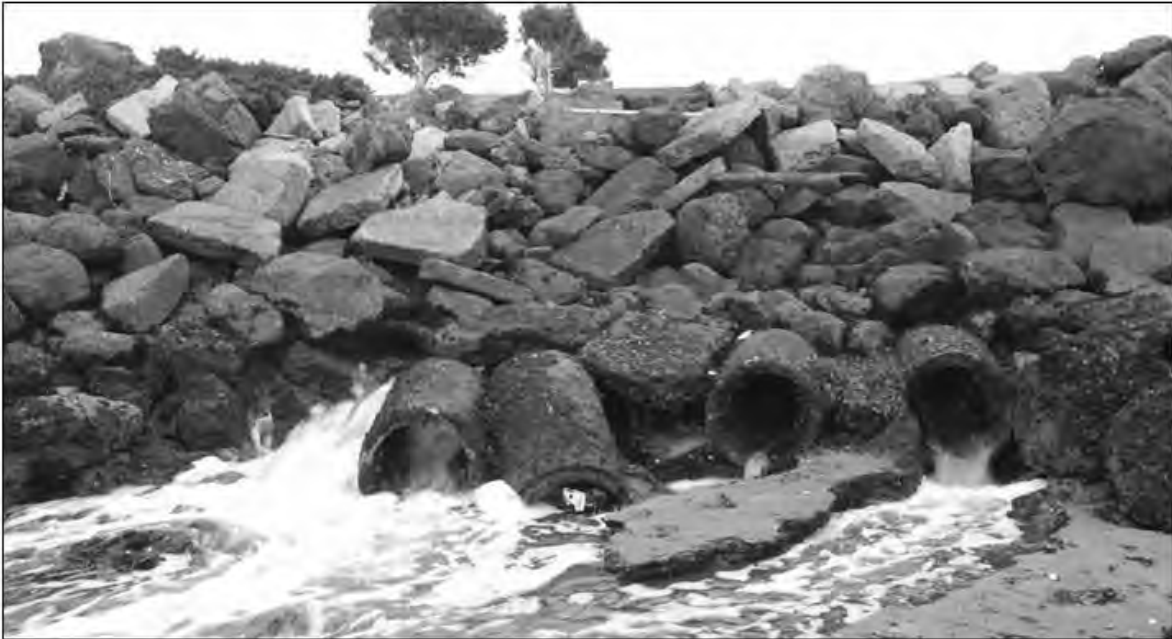
Broken Culvert Pipe Outfalls underneath I-80 at SF Bay shoreline : (Unstable shoreline slope, no wing wall protection, subsurface pipe failure is imminent)
